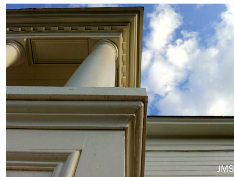
House No 3 is now fully restored. Call to reserve it for your next event: 541-374-8619
